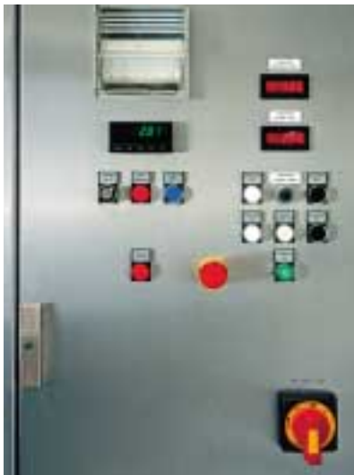
Operation panel with a clear indication of unit and process data
